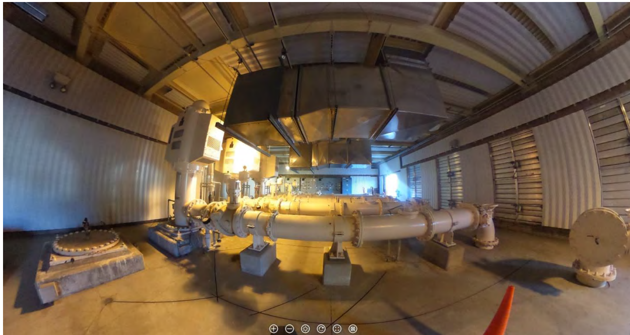
Figure 11-4: An Example 360-degree Photo Captured from Ogden Booster Pump Station
