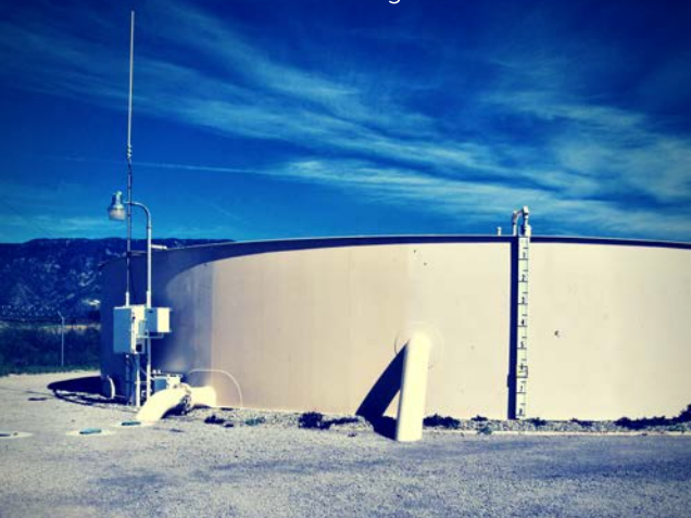
SBMWD Ridgeline Water Reservoir
