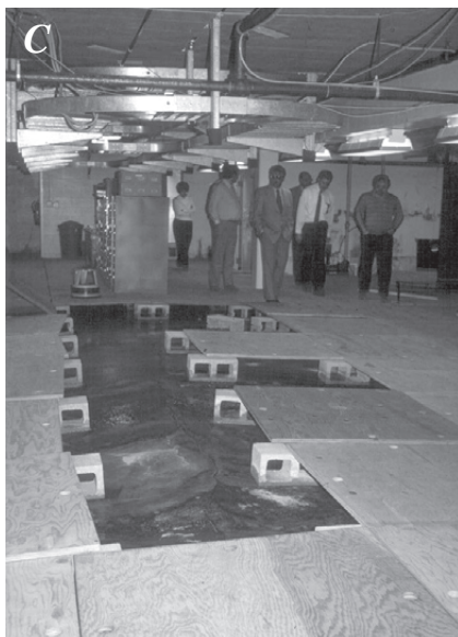
High ground-water levels in the former marshland. View shows groundwater upwelling through the buckled concrete basement floor of the San Bernardino Valley Municipal Water District, June 1985.
