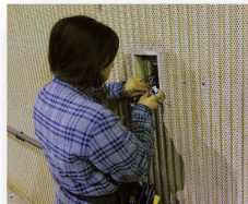
Electrical, Instrumentation, & SCADA
